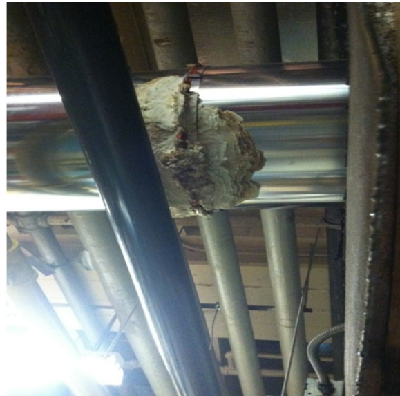
A leaking single-wall Special Gas Vent. The leaking condensate creates an ever-growing paste around the joint.
