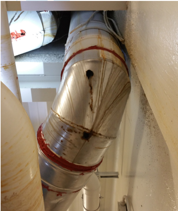
A leaking double-wall Special Gas Vent. Localised corrosion leading to perforation of the outer jacket.
